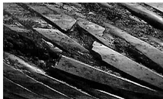
Cracks will propagate through the wire and result in breaks.
